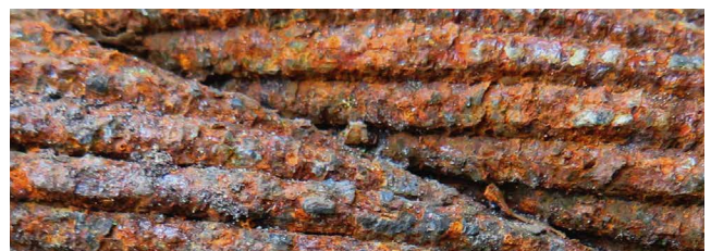
Enlargement of external corrosion
